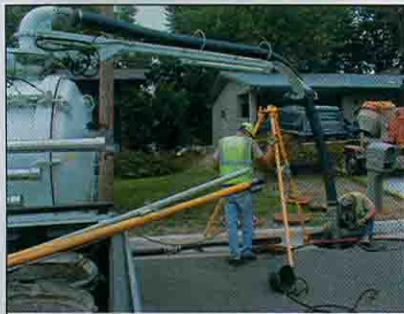
For ease of pump-out, access openings were located next to the curb.
